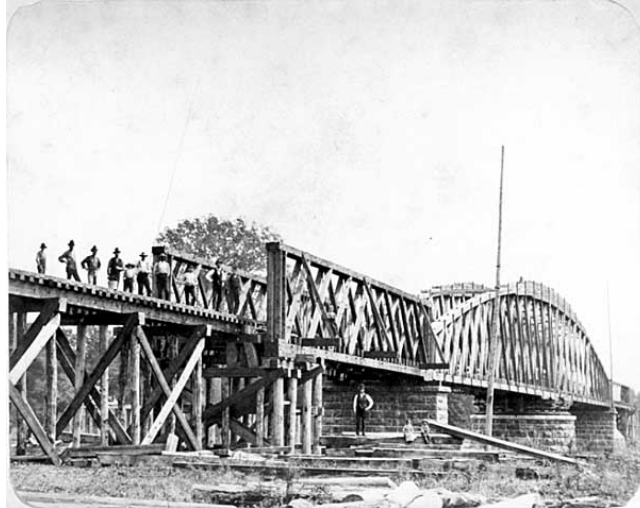
Building the Mpls. St. Louis Railroad's River Crossing Bridge at Carver, 1871 (mhs)
