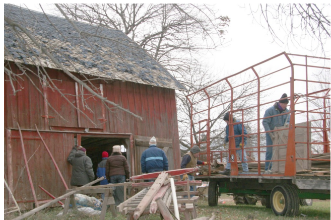
Commissioners Maluchnik and Workman along with the Nordic Group and CCHS work to save the north Andrew Peterson barn.
